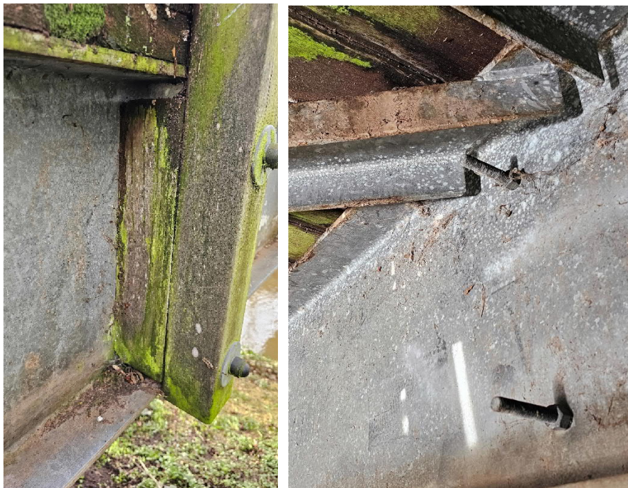
Figure 11: Parapet fixings showing nut on underside of bridge and spacer on outer face of girder.
