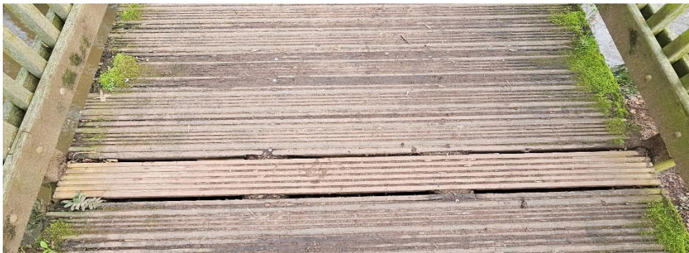
Figure 8: Deck surfacing showing unsuitable replacement boards.
