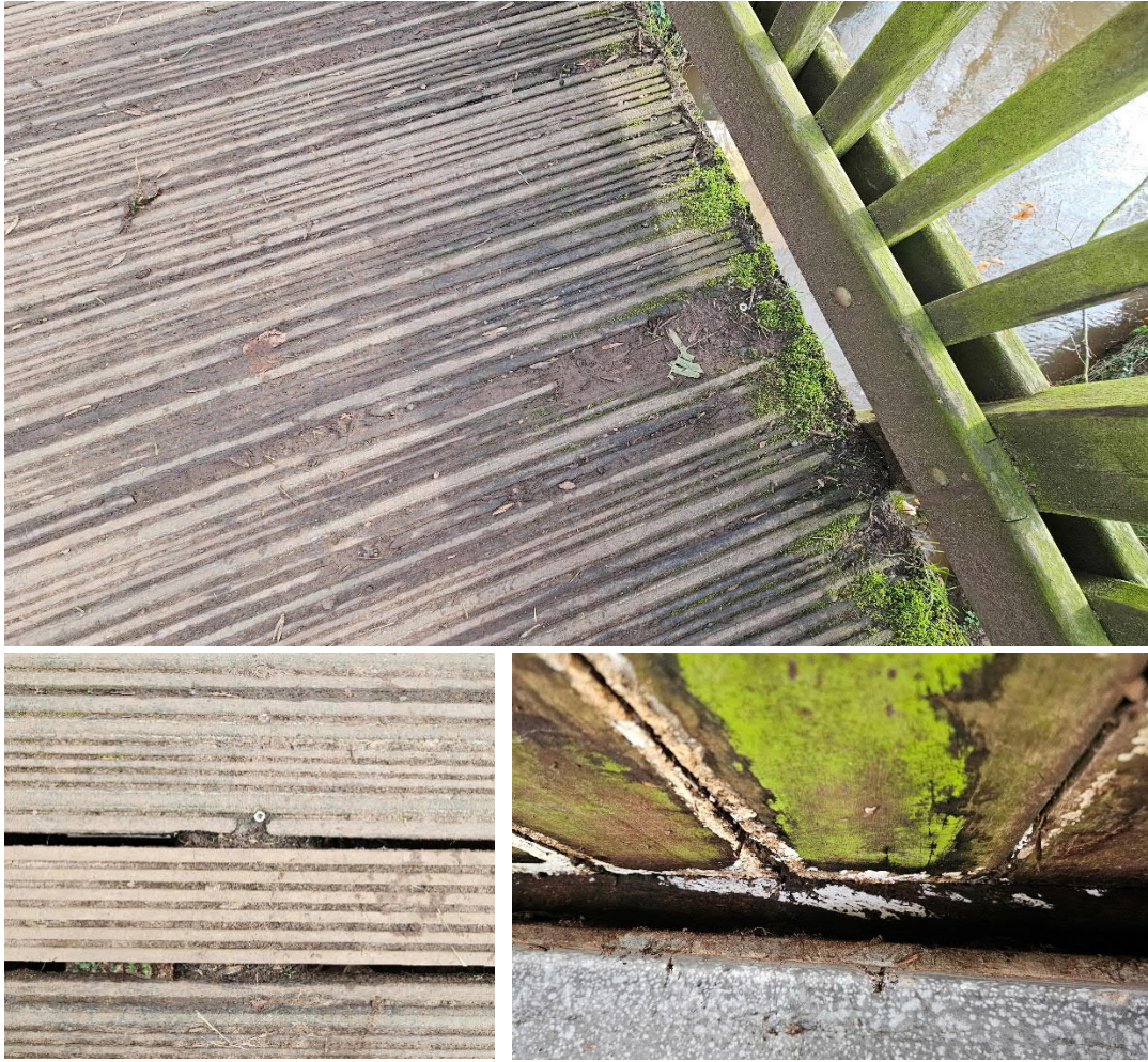
Figure 7: Deck surfacing showing decayed areas of boards.
