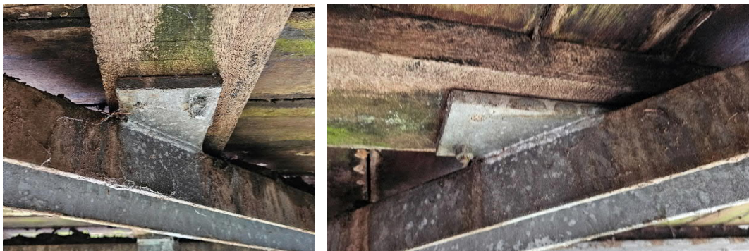
Figure 9: Deck board bearer locating fixings missing (example of).
